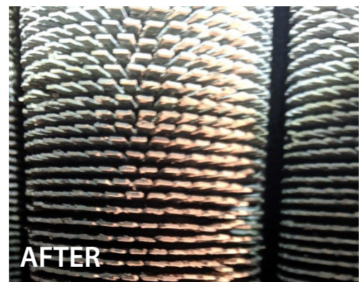
Finned tubes after EPIC cleaning.
