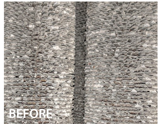
L.P. economizer deposits on finned tubes.
